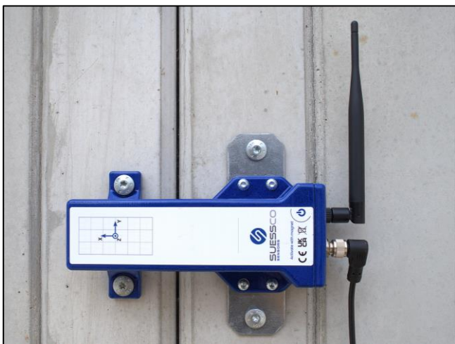
Reference crack application
